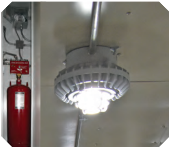
Fire Suppression System
